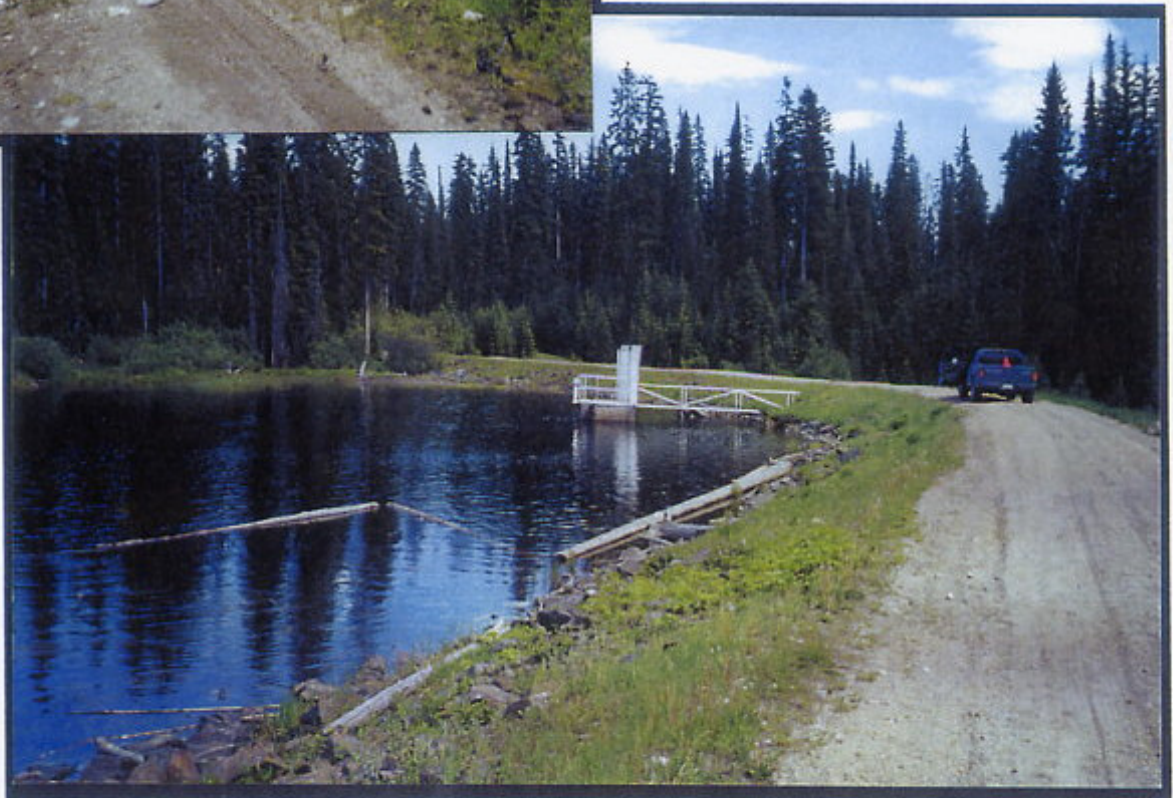
Tower Outlet Structure
