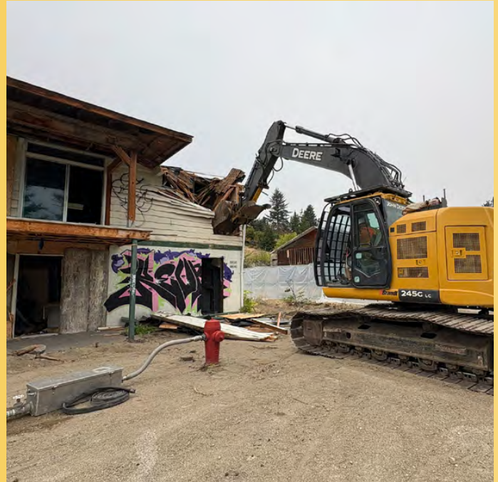
Airport Inn demolition – The 2025 demolition of the Airport Inn marked an important step in improving community well-being, with the removal of neglected buildings and bringing an opportunity for safer, cleaner, and more compliant development to the community.
