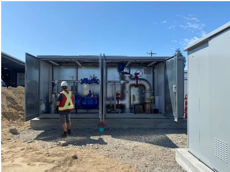
Figure 5 City of Kelowna Bulk Water Meter and PRV 24
