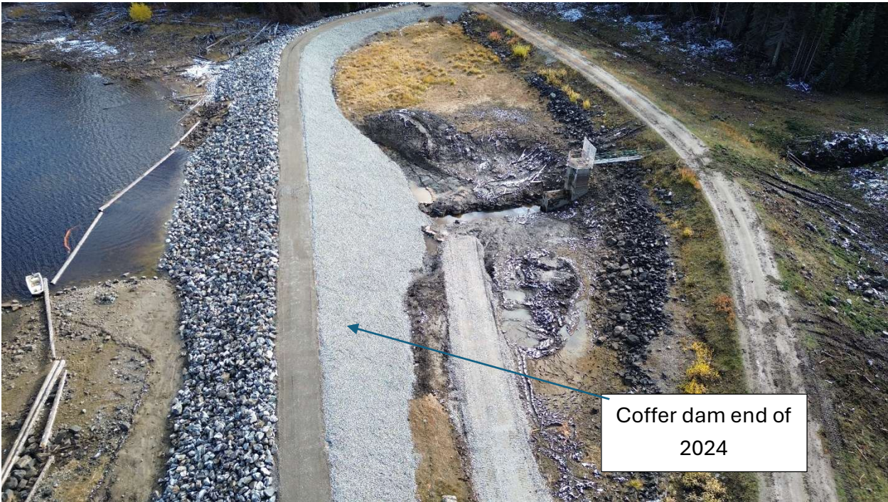
Figure 7 Aerial view of coffer dam holding back water in Beaver Lake to remove the old dam control structure
