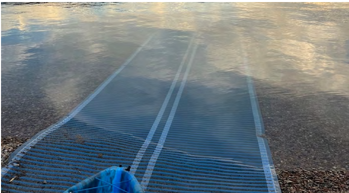
The newly installed Mobi-Mat leading from the pebbled beach into Okanagan Lake.
